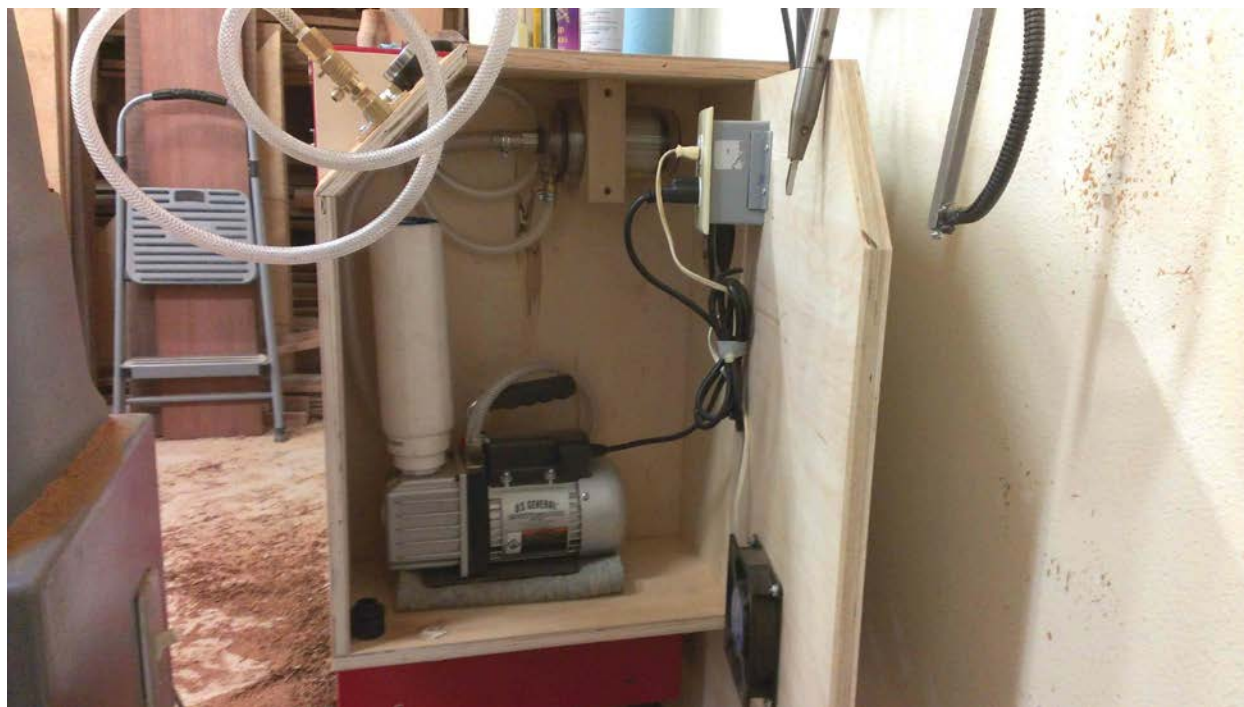
Figure 1. Filter in place on pump.
